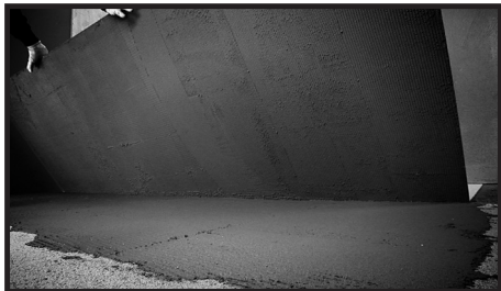
Fig.76 - Using these systems with big gauged porcelain tile 3000x1000 mm is complex (There is a potential risk of movement, and consequent mortar displacement, during the positioning of the gauged porcelain tile).
